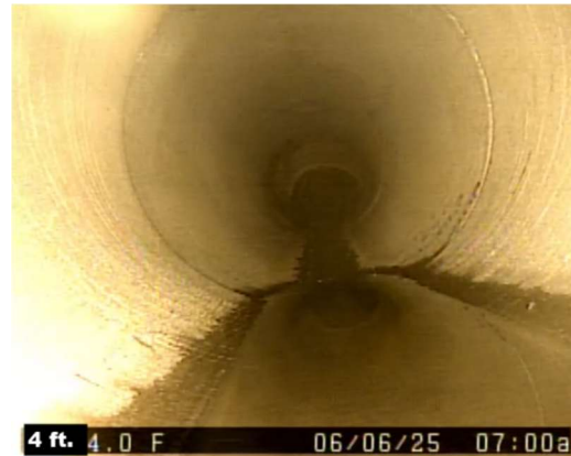
June 2025 storm sewer condition
