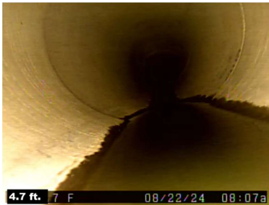
August 2024 storm sewer condition
