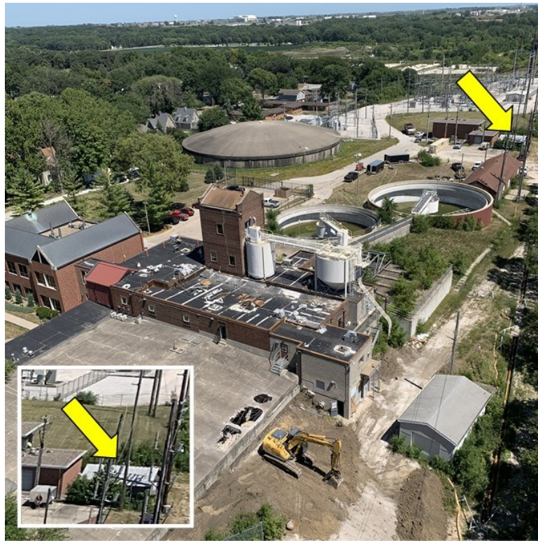
Photo (8-26-2022) of the old Water Treatment Plant at the start of demolition. The storage building with the unknown remnants of a pump station below is marked with an arrow.
