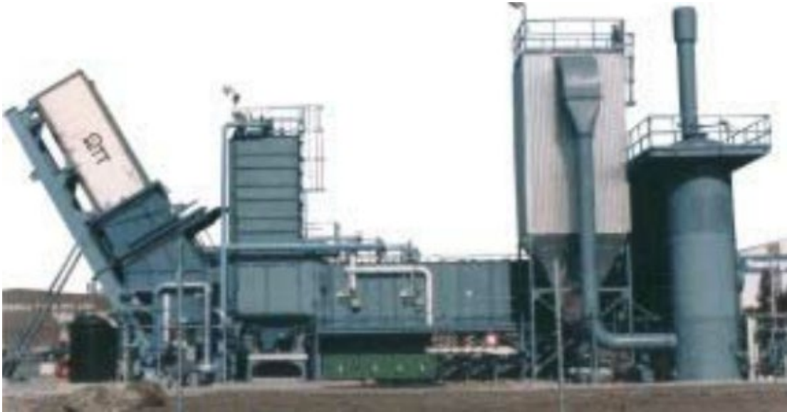
Figure G - 8: EnerSol Vibratory Hearth Combustion System
