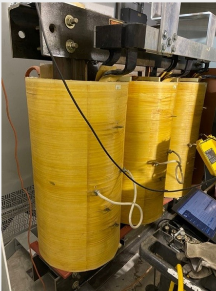
Pictured: Transformer testing and maintenance
