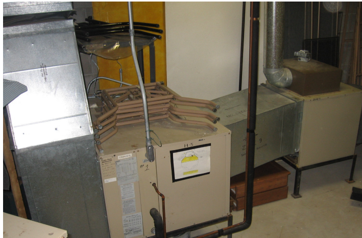
Blower coil and duct furnace serving one zone of the worship space
