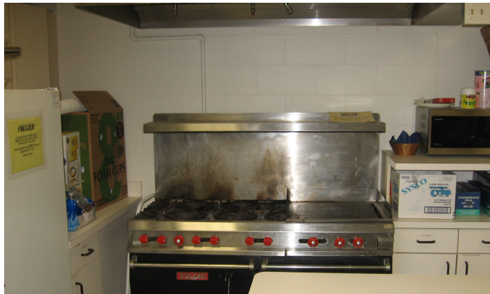
Kitchen range and exhaust hood located in the 1995 addition
