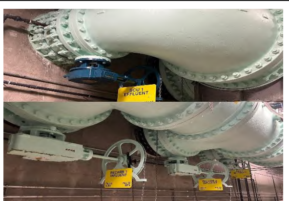
Solids Contact Unit and Recarbonation Valves. The manual chain wheel operators will be replaced with new mechanically actuated controls.
