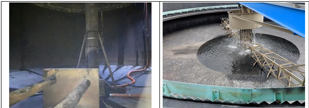
Interior of a primary digester during cleaning to improve performance and increase capacity.
