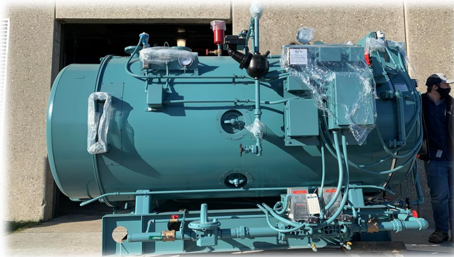
New dual-fuel boiler being delivered to WPC
