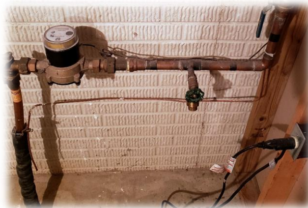
A typical residential water meter installation
