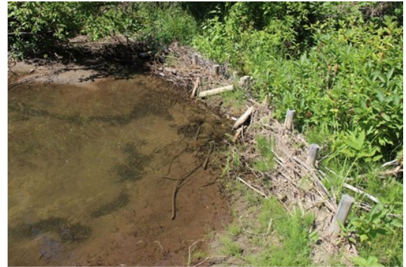
Figure 2. Installation of BDAs can take many forms, as different structures shapes, sizes and locations can be designed to promote specific outcomes at the structure scale. Building a diversity of structure types accommodates variability and uncertainty in stream flows and is more likely to encourage the recovery of degraded processes (e.g., erosion, deposition, overbank flow) that are crucial to meeting restoration
