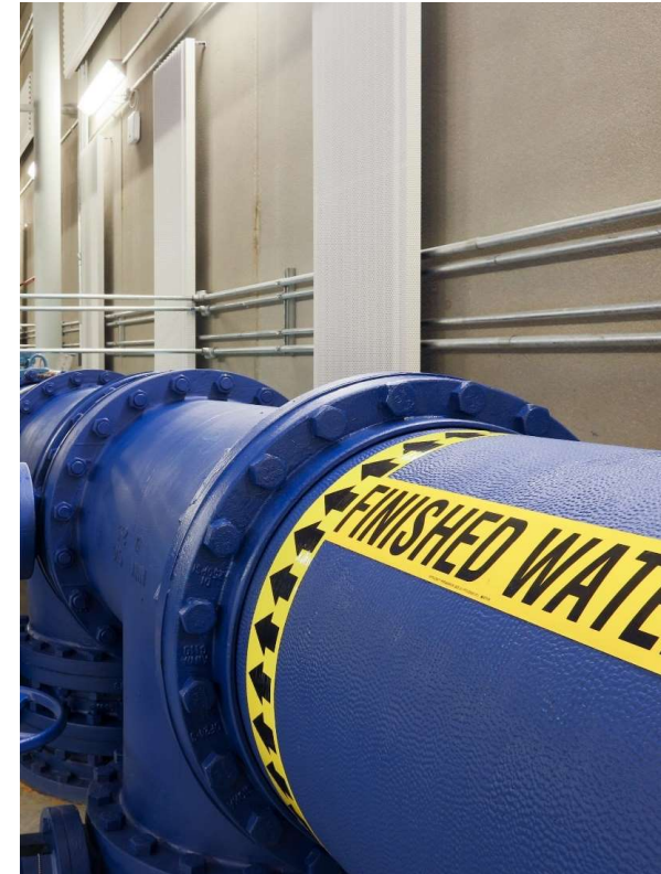
Piping in High Service Pump Room Ames Water Plant
