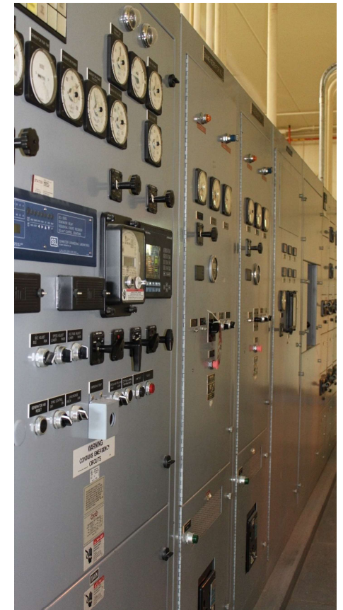
Cogeneration switchgear Ames Water Pollution Control Facility
