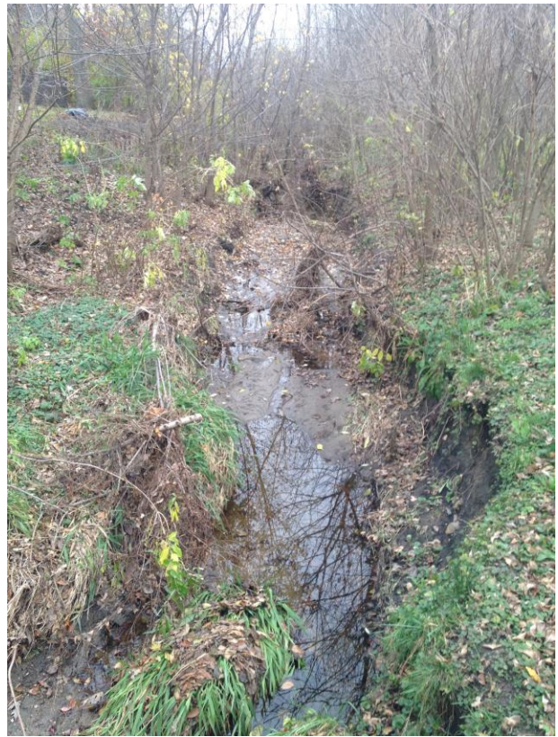
Channel degradation upstream of Hoover Avenue/Edgewater Drive.
